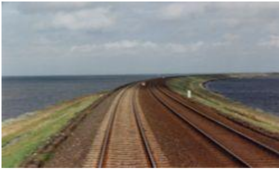
The rail causeway across the Wadden Sea to the island of Sylt in Germany
