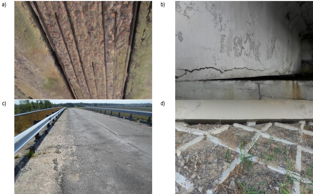
a) thawing (frost destruction) of concrete with bare and corroded reinforcement; b) corrosion cracks (corrosion of principal reinforcement); c) patching in the bridge deck covering; d) cone subsidence under the end piers nozzles
