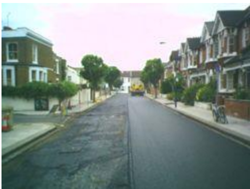
A road in the process of being resurfaced, showing both old and new asphalt surfaces.
