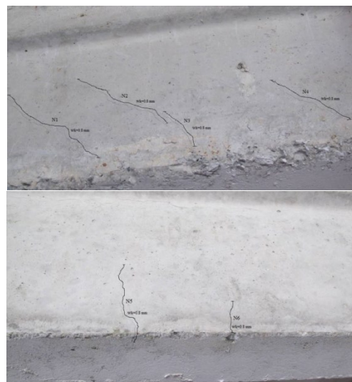
Figure 12 – Characteristic defects of the evaluated precast beam and ribbed slabs
