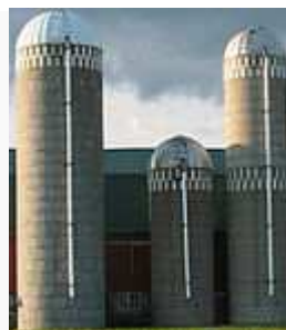
Small stave silos can be expanded upward. More hoops are added to strengthen the lower staves.
